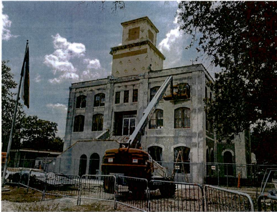
1- Date Taken: 8/24/2023 Taken By: A. Skellie Exterior Overview: No visible loss related damages.
