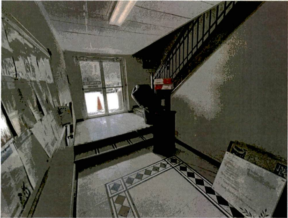
3- Date Taken: 8/24/2023 Taken By: A. Skellie Hallway Overview: Damages to bottom of walls and flooring.
